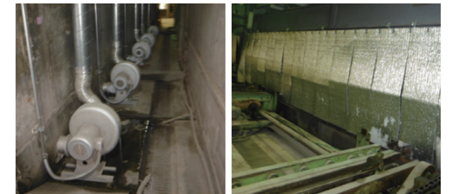
Air distribution fan (left) and heat retention curtain (right) newly installed to stabilize temperature inside curing chamber
